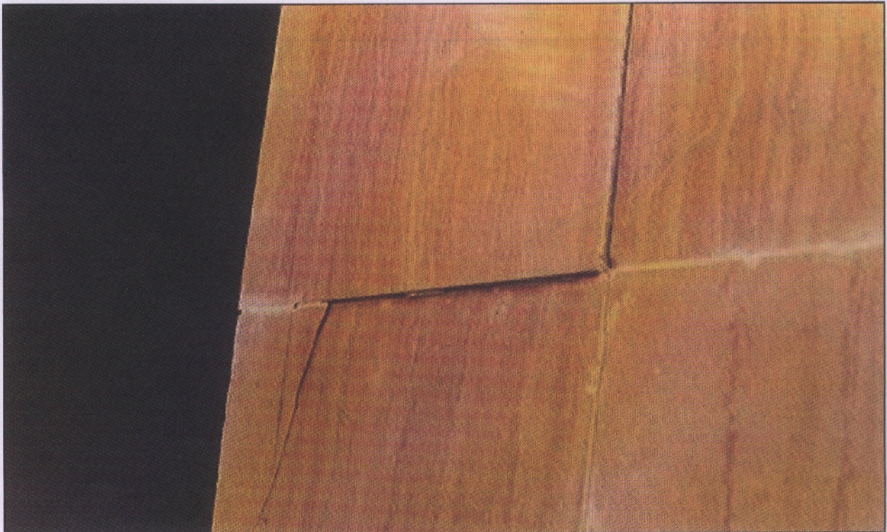
Marble cracks due to settlement
