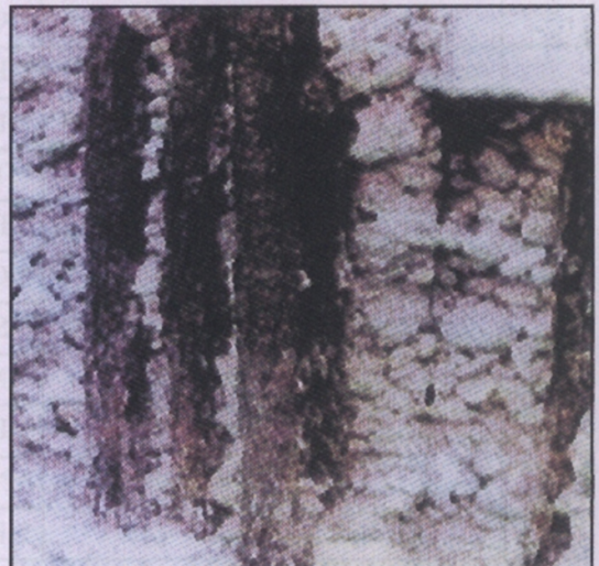
C2 - Close up of corroded reinforcement
